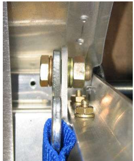
Photo 11 Outboard Attach Point Detail
