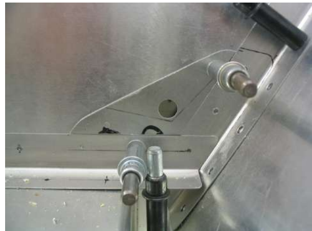
Photo 6 Shim for 6B18-3 Attachment Doubler Plate
